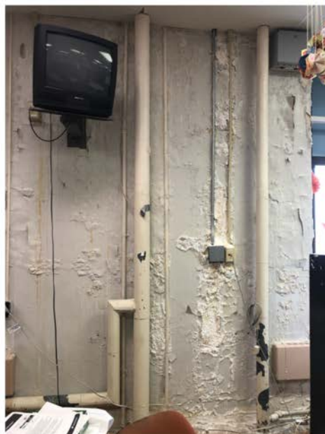
Left: IMC/Library Submitted: April 30, 2021 Last District Update: June 9, 2021- All paint and plaster issues are currently being checked by maintenance personnel on the best way to address this situation
