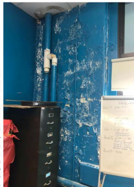
Right: Room 106 Submitted: Repeatedly over the course of years. First report 9/4/2019. Last submission from April 2021, with note: Twice fixed, paint flakes and turns into dust when the window is open. Last District Update-1: September 27, 2019: Work order created for Painters Last District Update-2: June 9, 2021: All paint and plaster issues are currently being checked by maintenance personnel on the best way to address this situation
