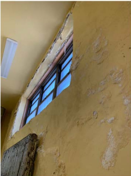
Left: Room 300 Submitted: October 2, 2019 Last District Update: December 3, 2019- Work order created for plasterers
