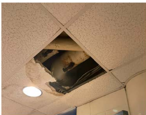
Above: Outside Cafeteria Submitted: September 27, 2021 Last District Update: October 13, 2021- Tile has been cut to remove mold, light is supported by rest of tile, if remaining tile is removed light will have to be disconnected
