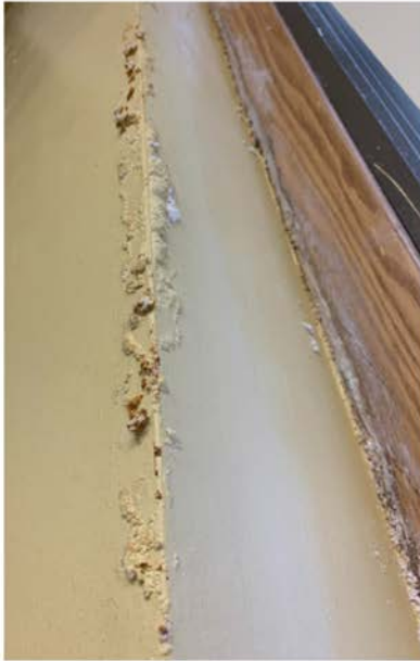
Left: Room 304 Submitted: October 7, 2019 Last update from District: October 27, 2019- Work order created for plasterers
