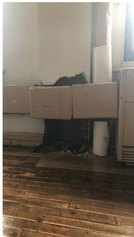
Right: Room 320 Submitted: April 30, 2021 Last District Update: June 9, 2021- All paint and plaster issues are currently being checked by maintenance personnel on the best way to address this situation
